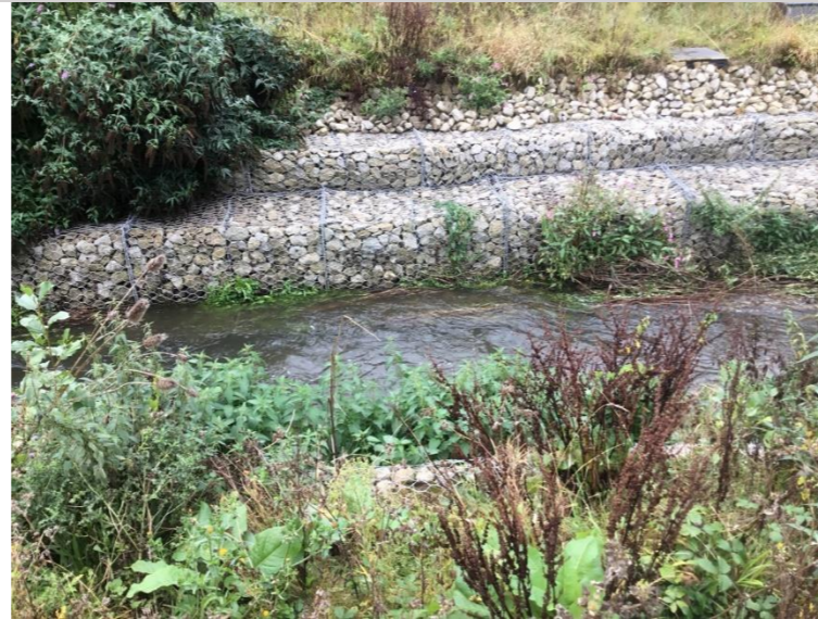
Photo 60: Gabion rock baskets provide bank protection on left bank due to scour at nick point in channel
