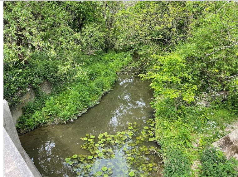
Photo 34: Channel downstream of London Road bridge, berms formed at margins
