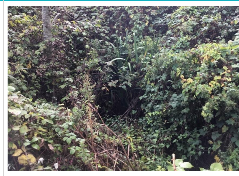
Photo 114: Culvert outlet heavily vegetated
