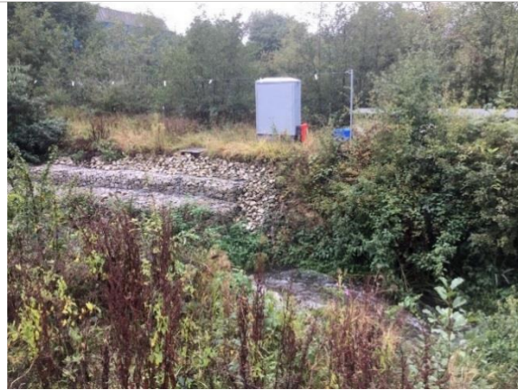
Photo 3: Gabion mattresses and erosion of bank
