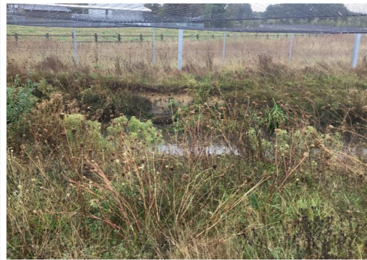
Photo 54: Localised bank erosion of steep banks and slumping of material
