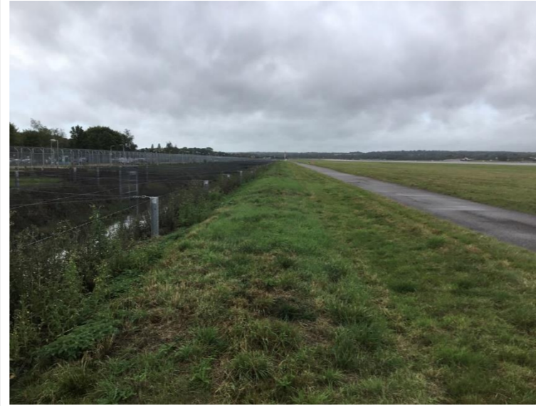
Photo 104: Low embankment on right bank with small breaks
