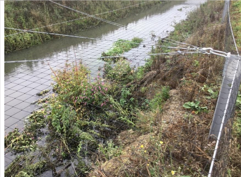
Photo 97: Bank erosion and slumping of material into channel
