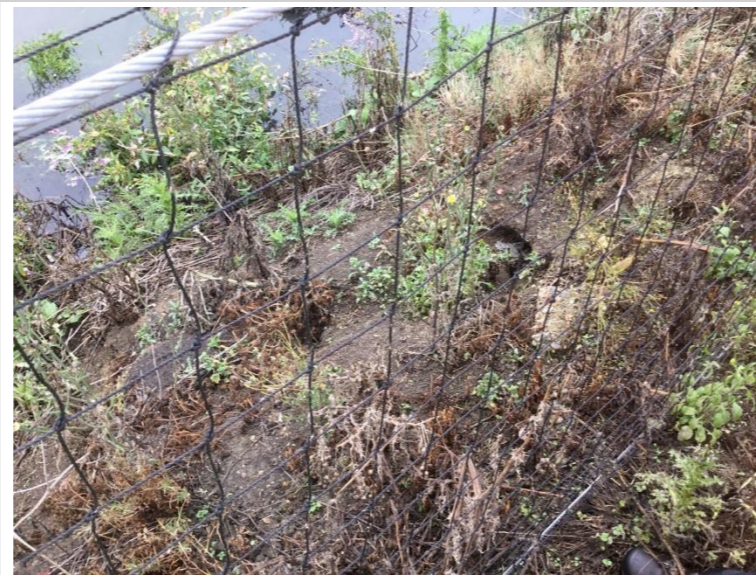
Photo 98: Animal burrowing in failed banks
