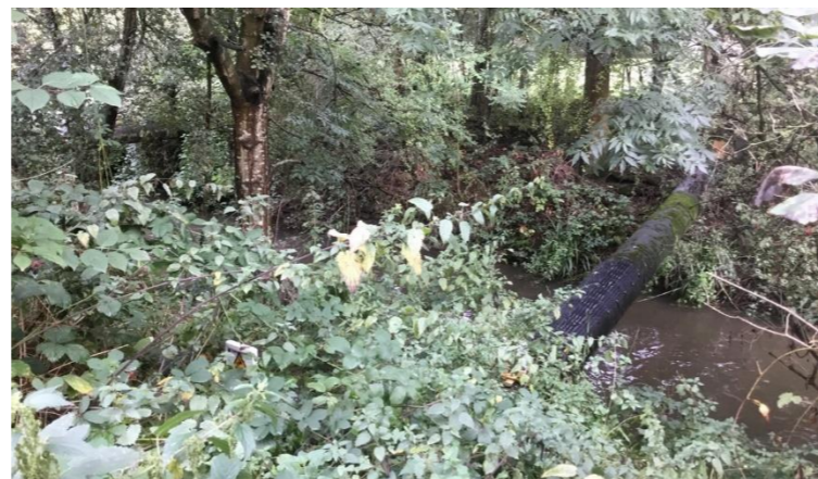
Photo 70: Several pipe crossings over Gatwick Stream
