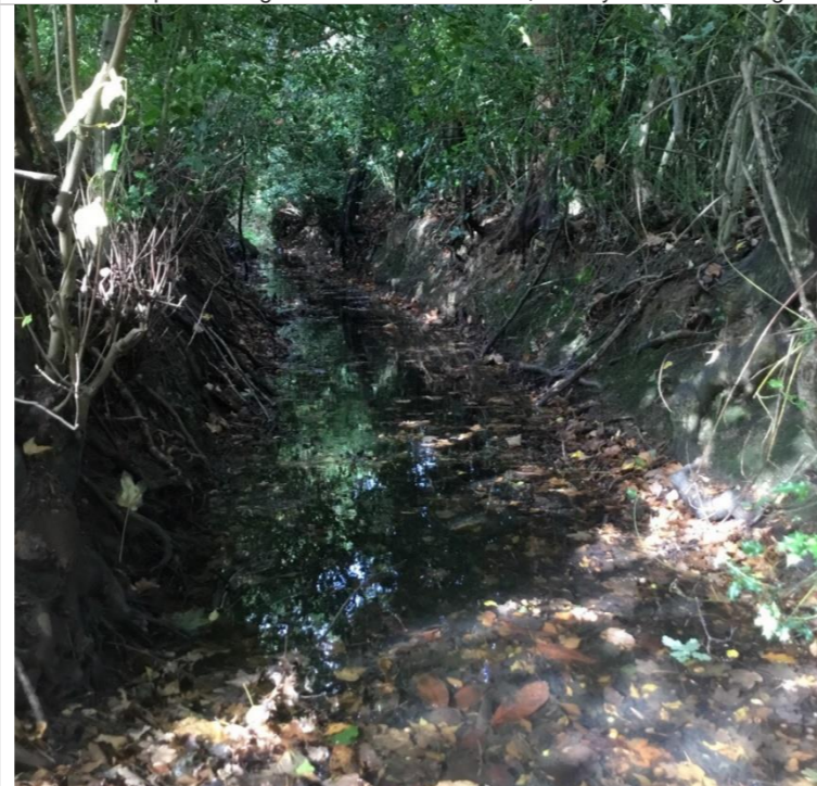
Photo 116: Downstream of culvert along Balcombe Road, heavily shaded, no perceptible flow. Organic material including leaf litter on bed.
