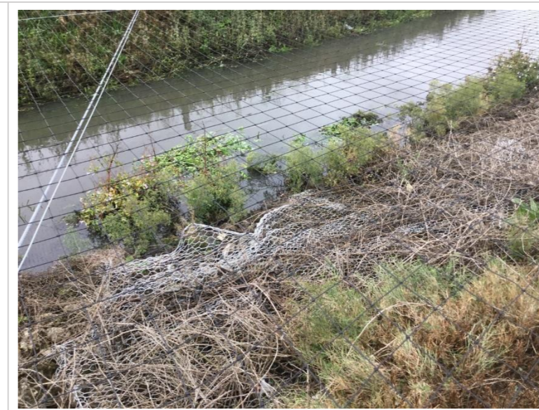
Photo 96: Damaged gabion mattresses, evidence of high discharge damaging defences
