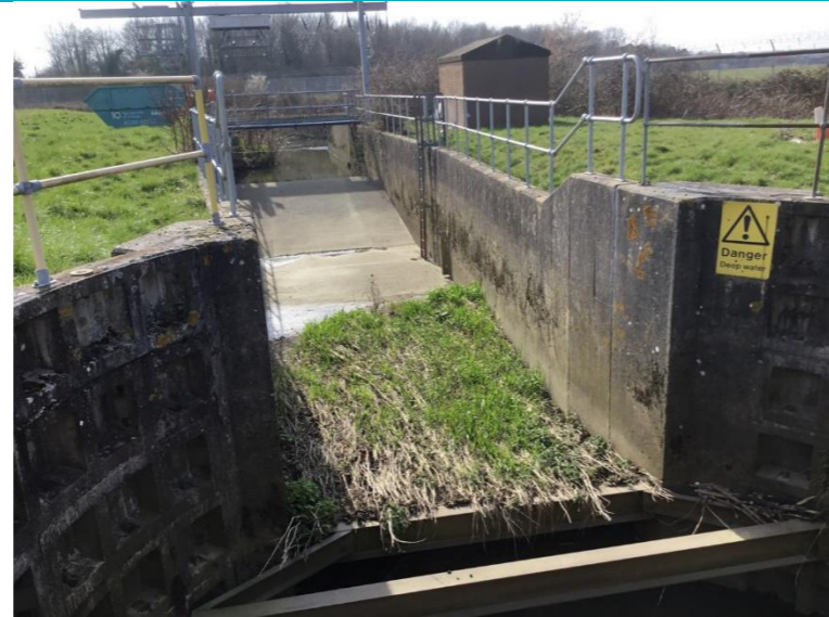
Photo 2: Syphon channel from River Mole and gravel accumulation next to drop chamber
