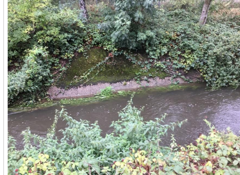
Photo 58: Channel is concrete lined from railway downstream along straightened section to footpath bridge
