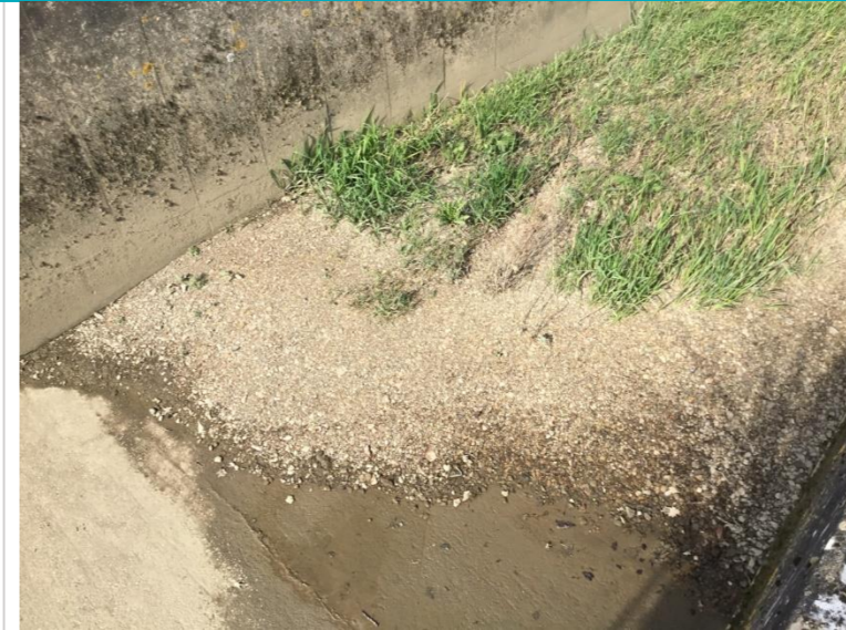
Photo 3: Fine to medium sized gravel accumulated on syphon channel
