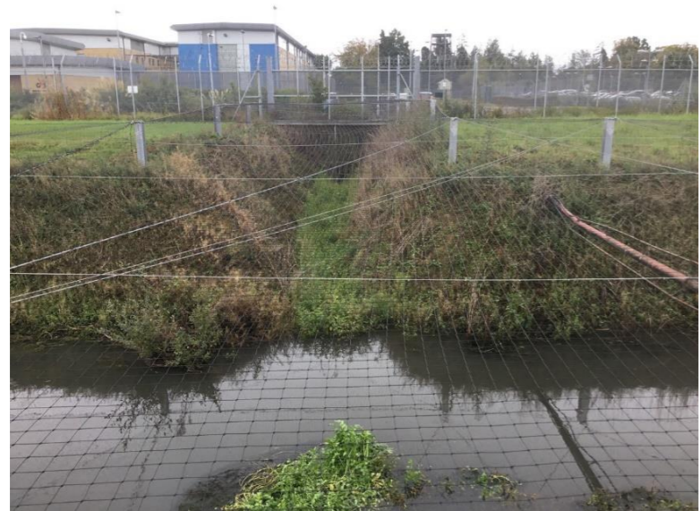
Photo 103: Concrete outfall and vegetated spillway
